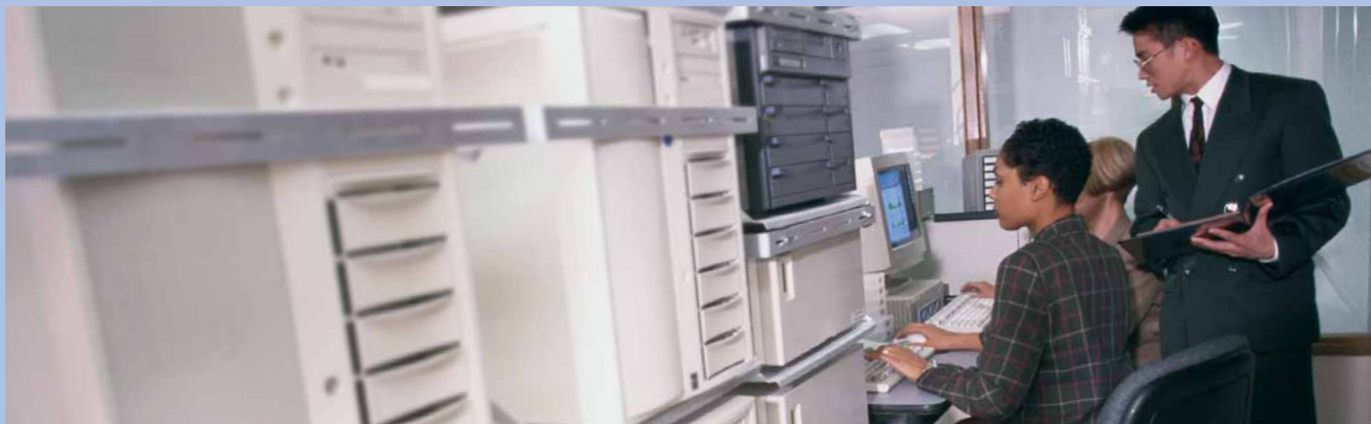
Data centre: Security application
